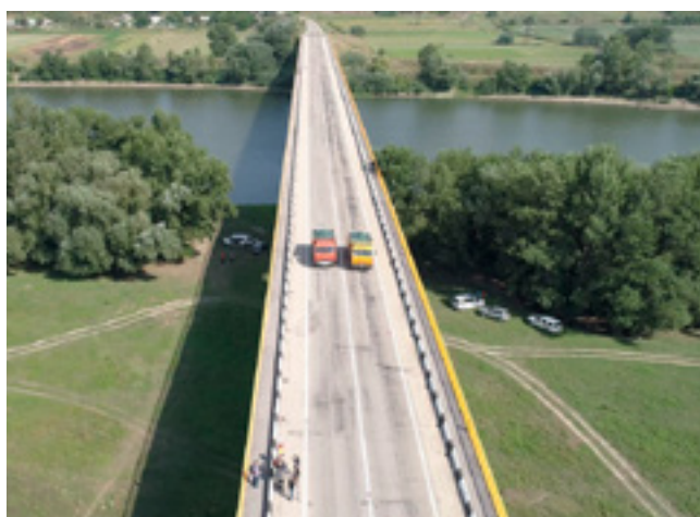
Technical assessment works ongoing on the bridge between the villages of Gura Bicului and Bychok, which is part of an international transport corridor linking Moldova to the port of Odesa and to the European Union. (OSCE)
