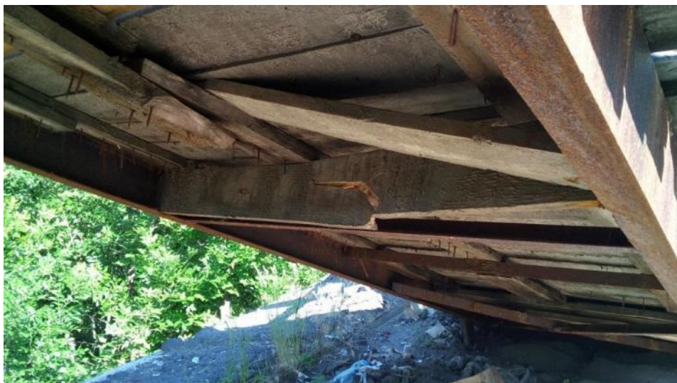
Damage to Stanytsia Luhanska bridge wooden ramp observed on 21 June
