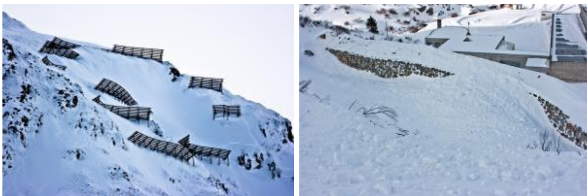
Figure 10, left: Metal barriers installed in the avalanche starting zone threatening the entrance to the tunnel. Right: Retaining wall constructed in the runout zone above the entrance to the tunnel.
