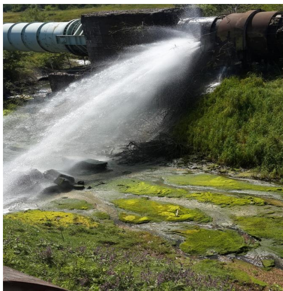
Figure 2: Damaged water pipeline near Horlivka
